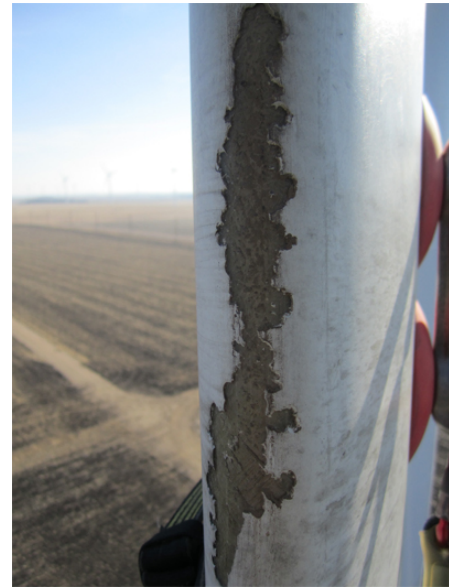
Figure 1: Wind Turbine leading edge erosion affects aerodynamic performance and structural integrity of the blades.
