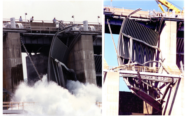
Figure 2: 87-ton Tainter-gate failure at Folsom Dam in USA, on July 17, 1995.
